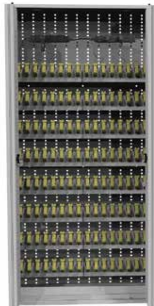
128 Taser Storage using Bi-Fold Security Cabinet with charging unit
